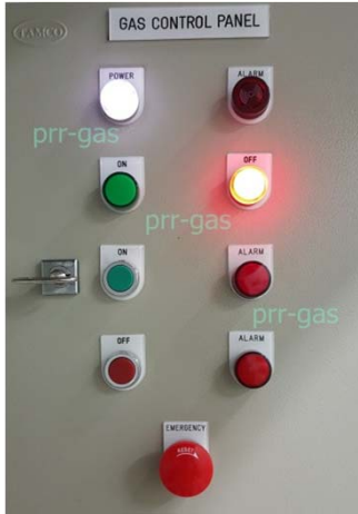
Cas Control Panel
